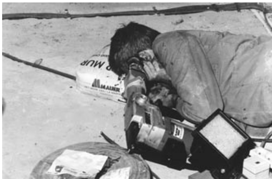
FIG. 1—Man found dead lying on the floor of a construction site, holding a pneumatic hammer.
